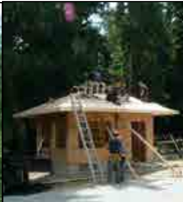
A new facilities block for the railway, built by the students at the local building trades college with materials provided by VIME. This just seemed to be such a marvelous initiative, especially as most model engineers these days are showing their age.
